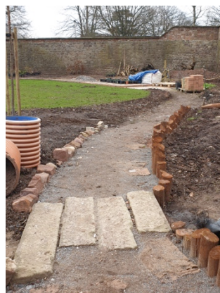
Left: A simple stone bridge crossing over our dry river bed. Made from what might have been heavy window ledges or lintels that we found buried in the garden.
